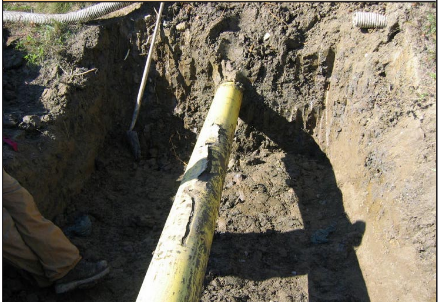
Coating Damage Identified by ECDA Survey
